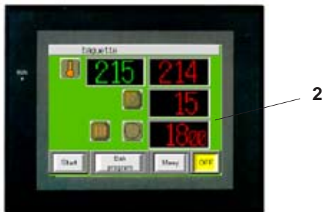
BCS-Baking Control System
