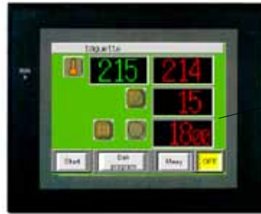
BCS-Baking Control System
